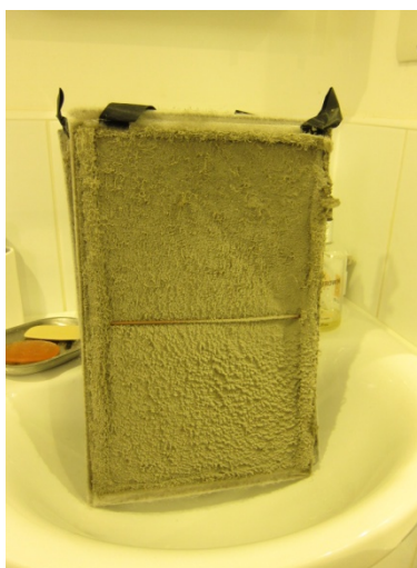
Figure 24 – Gap in Connection between Flexible Ducting in Dwelling B
