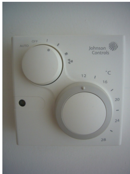
Figure 6 – MVHR and Heating Controls in Dwelling
