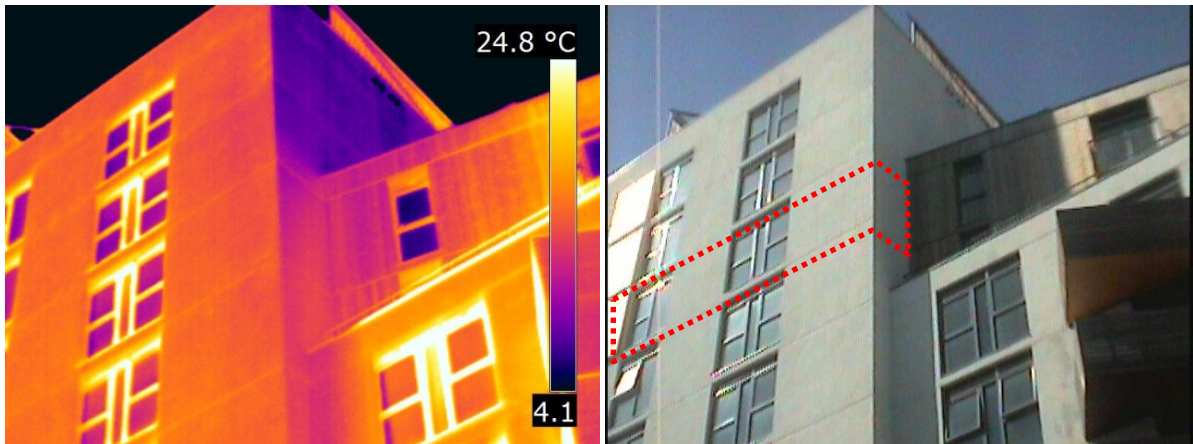
Figure 17 – Thermogram and Photograph of South East Wall of Co-heating Test Dwelling
