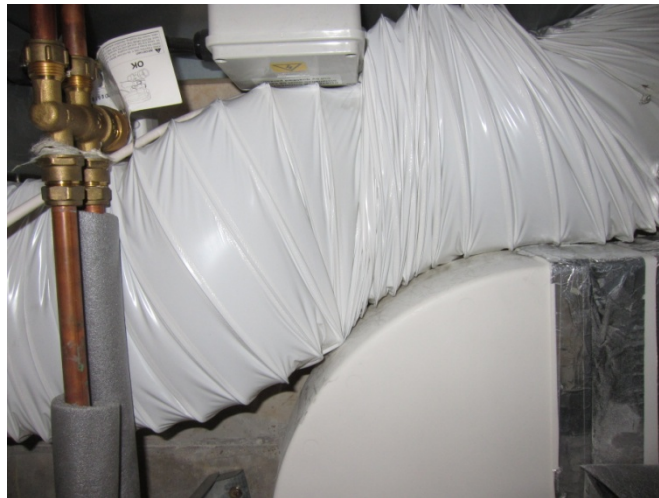
Figure 26 – Fat Deposit on Kitchen Air Valve
