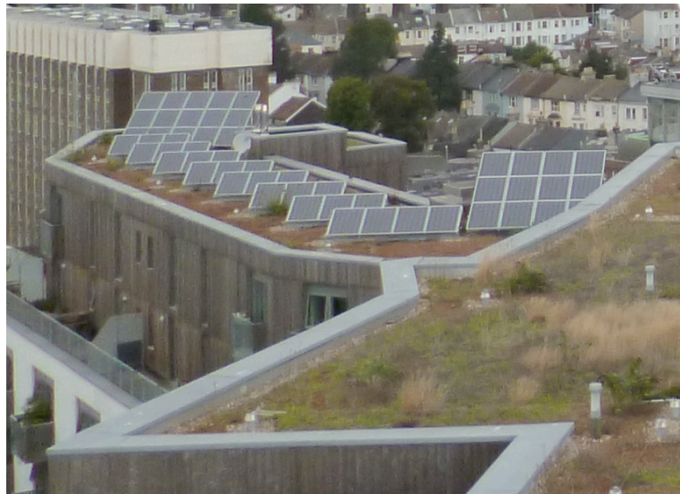
Figure 75 – PV Array on Roof of Pullman Haul Building at One Brighton
