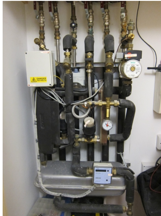
Figure 4 – Heat Interface Unit
