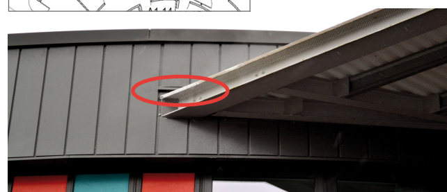
Figure 7.1: Location of leakage found in the rotunda during the smoke box test.
