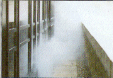
Tests revealed Gardner House to have an air leakage rate of 27 m 3 /h/m 2 at 50 Pa.
