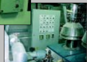
...but thumbs down for placing the summer/winter switch at the end of a plantroom obstacle course.
