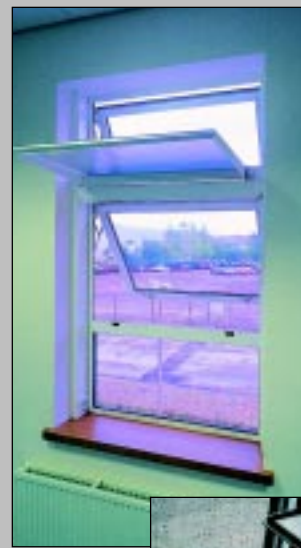
Occupants liked the upper motorised window, but the central window elements close under only a small wind, leading to...
